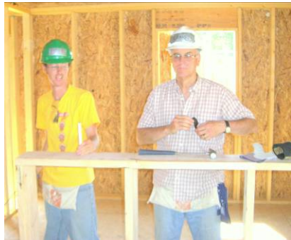
Craig Eley , and son Paul, building a half-wall and looking for some help!
