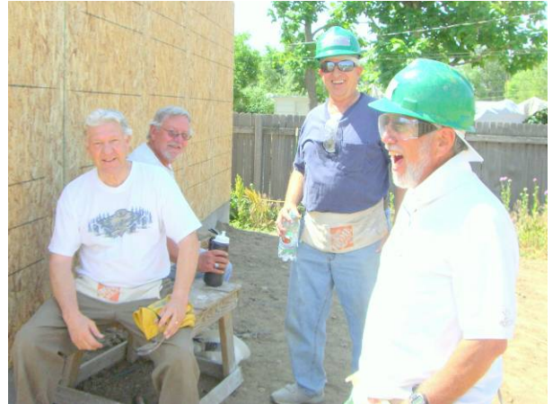
Here's the HELP taking a break: Oscar Sorensen , O.C. Larson , Jim Rumer and Ed Collins . They claim to be building part of a garage.
